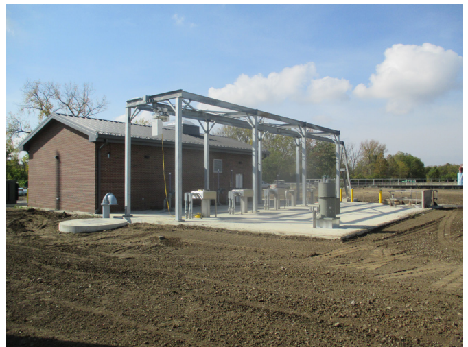
Glosser Road Pump Station & Columbia Road Booster
